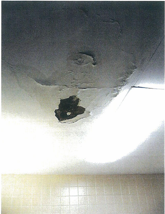
Wilber Hall - Men's Toilet Third Floor - Ceiling
