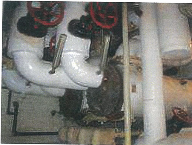
Wilber Hall - Distribution Piping
