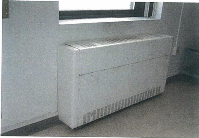
Wilber Hall - Unit Ventilators
