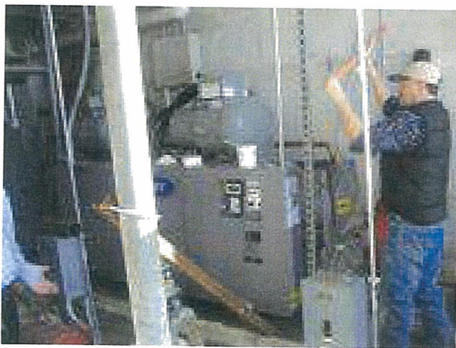
Wilber Hall - Chiller and Cooling Tower
