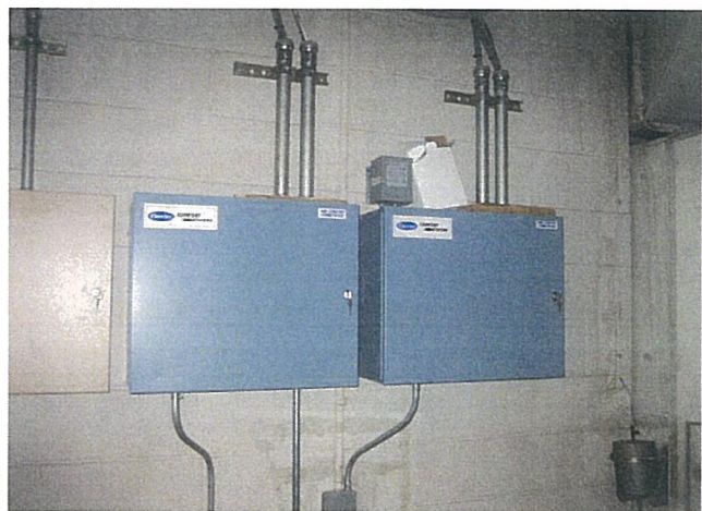
Wilber Hall - Pneumatic System
