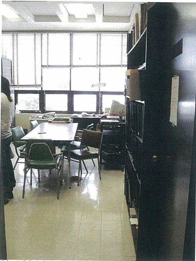
Mahar Hall, Typical Minor Water Damage
