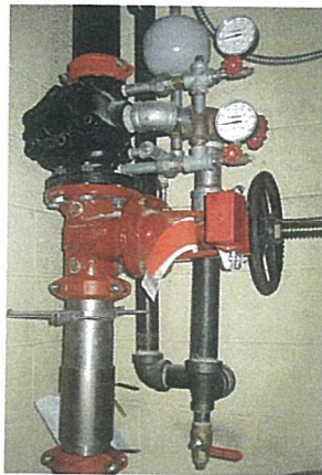
Wilber Hall - Fire Valves
