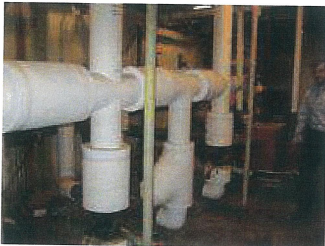
Wilber Hall - Distribution Piping
