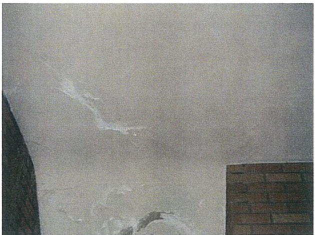
Wilber Hall - Penthouse Water Damage
